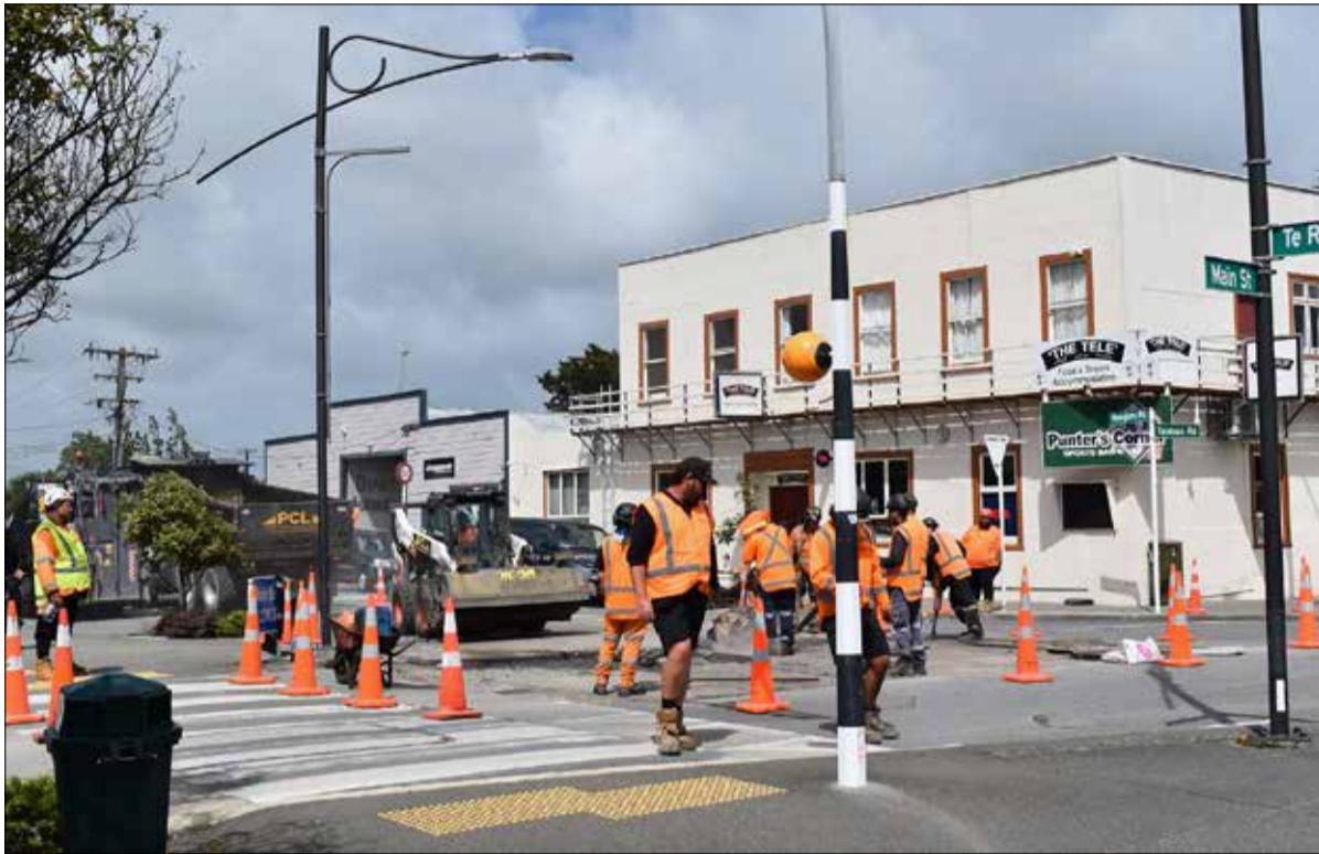
Workers at the Rangiuuru Road intersection, part two of an upgrade of the road surface and pedestrian crossings.
